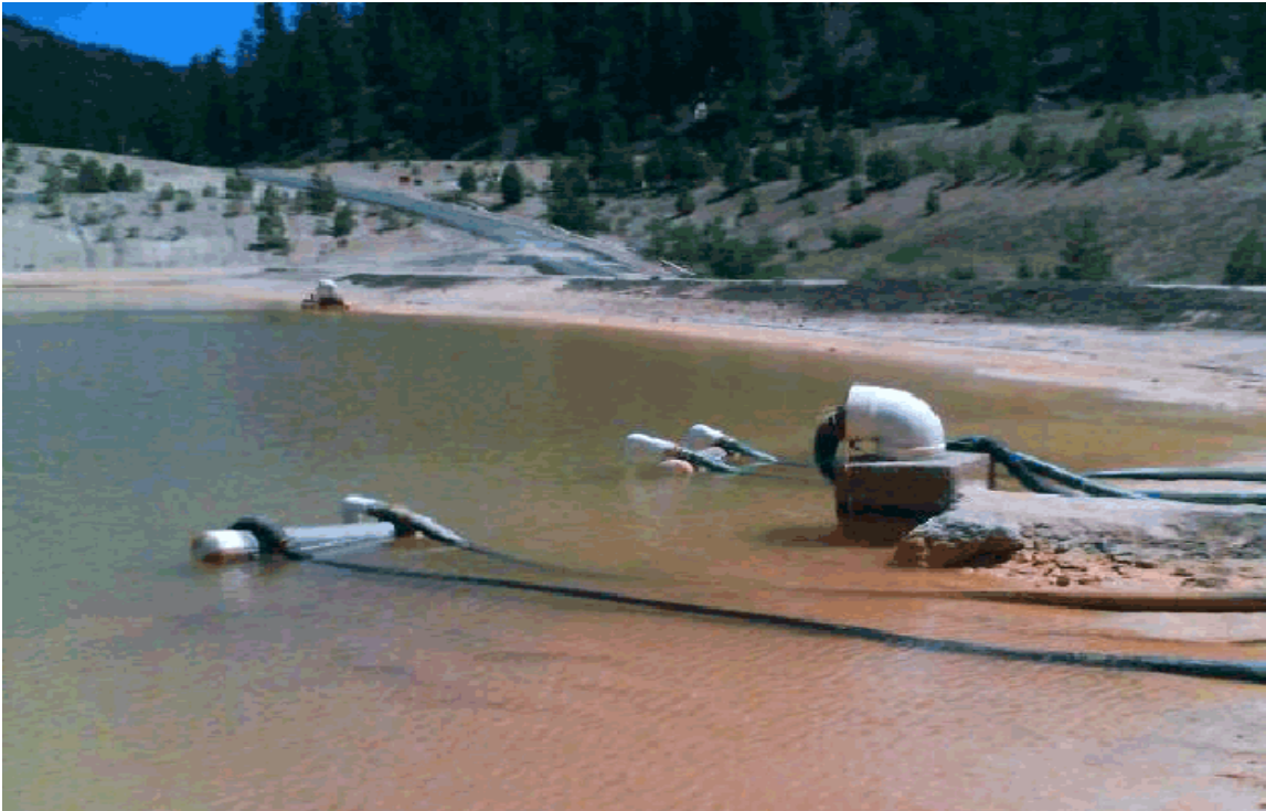
Figure 3 Suction lines located near surface to avoid discharge of sediments.
