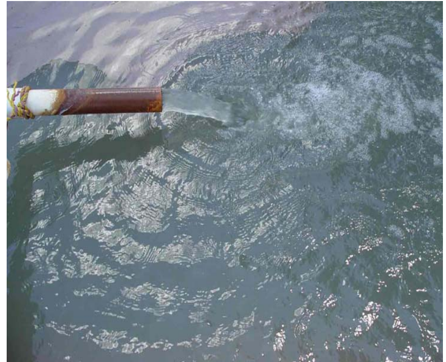
Inflow bioreactor 1. Low metals, high sulfates.
