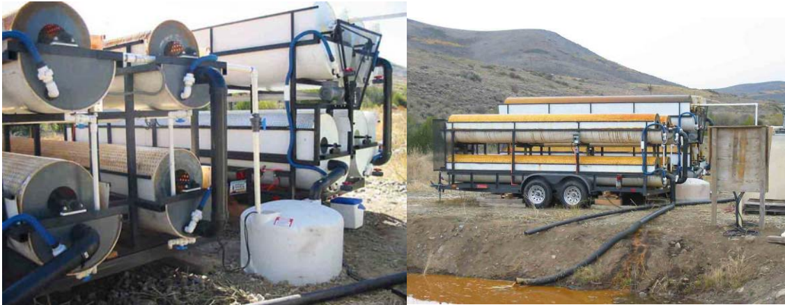
Figure1. The 600 gallon capacity and 1200 gallon capacity units at the Rio Tinto Mine Site
